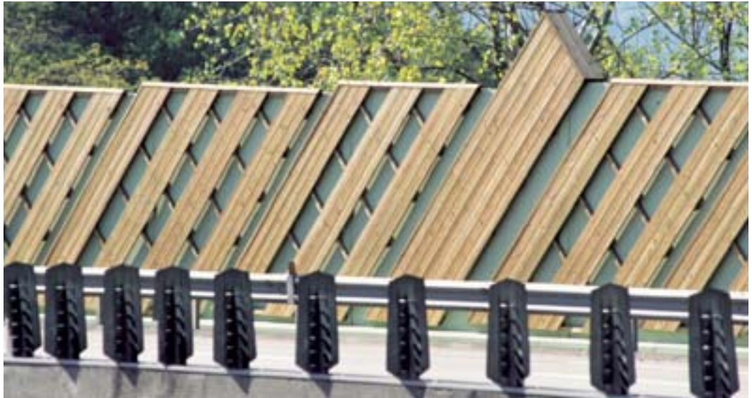
Noise barrier on the A7.
